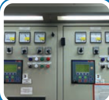
Gen Set Engines Testing
