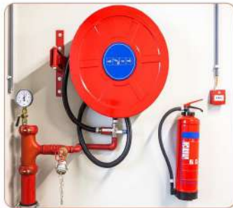
FIRE HOSE REEL
