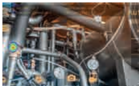
Compressed Air Leak
