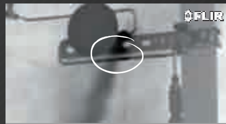
A LEAKING PRESSURE GAUGE
