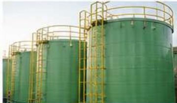
CHEMICAL STORAGE TANKS
