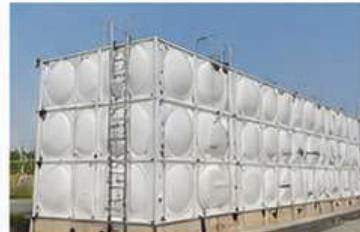
WATER STORAGE TANKS
