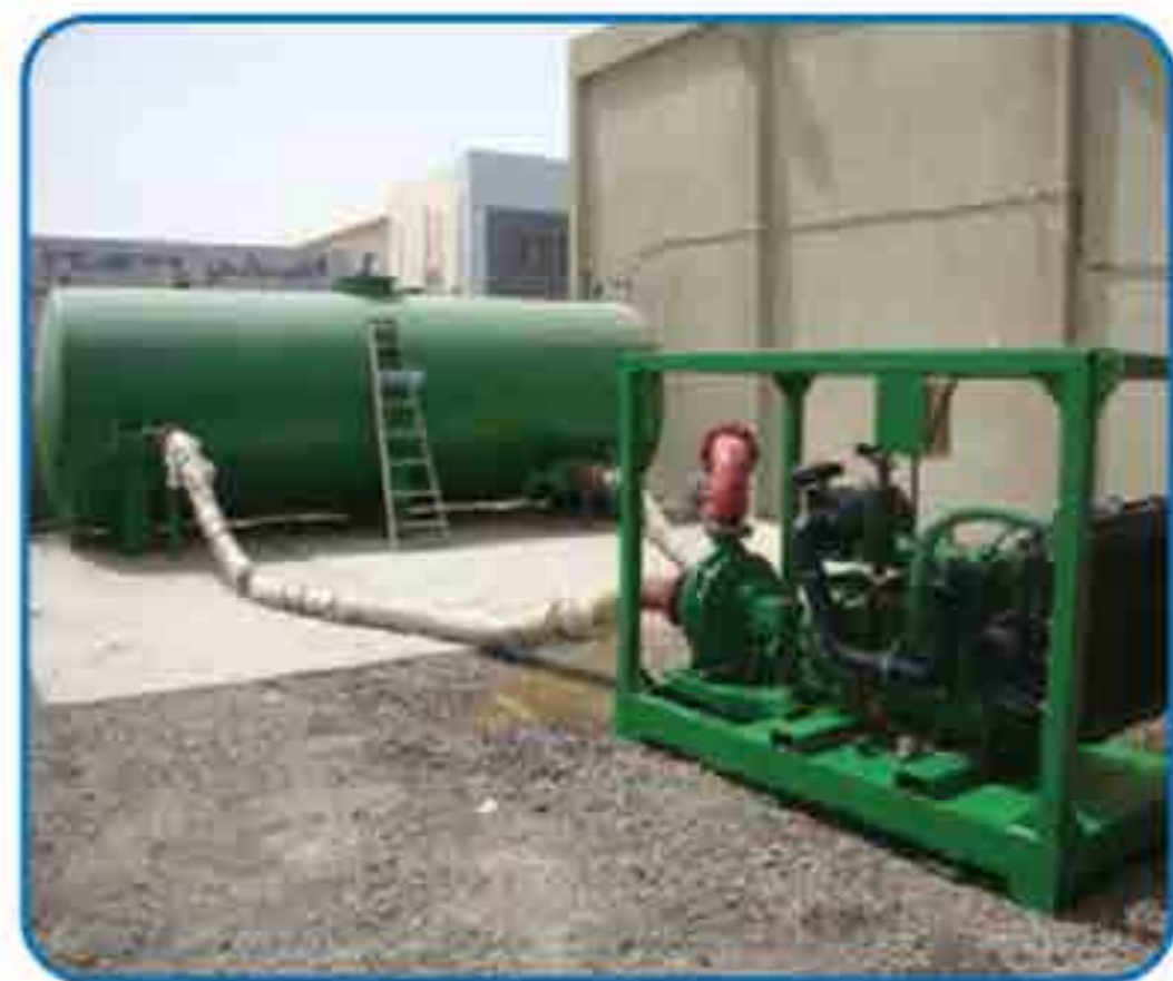
Diesel driven centrifugal pump on test
