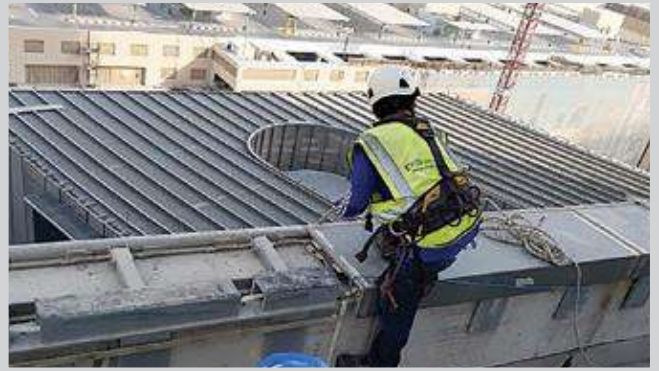
Facade Light Fixing
