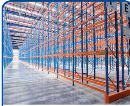
Selective Pallet Racking
