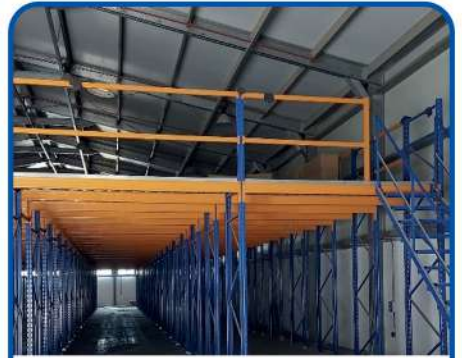
Rack Supported Mezzanine
