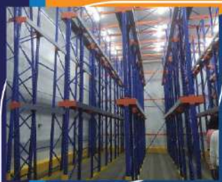
DRIVE IN RACK
