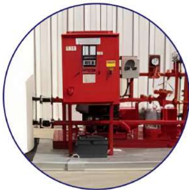
Diesel Pump Skids
