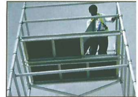
Trap Door Access.
