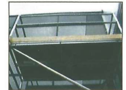
Platform With a wind Security System (to protect against Strong Updrafts)
