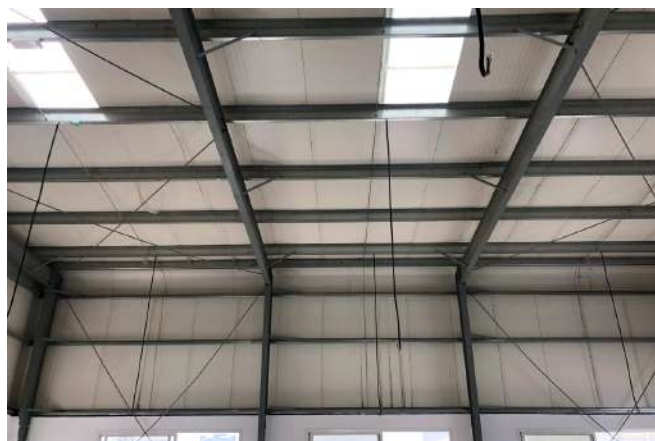
TRANSLUCENT ROOF LIGHTING
