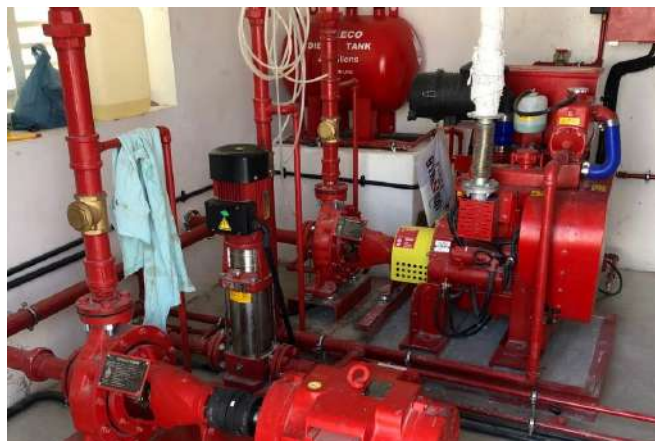
FIRE PUMP ROOM — COMMISSIONED
