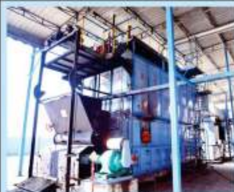
Jadeed Feeds Shakhkot (10 TPH Coal Fired Chain Grate steam boiler)
