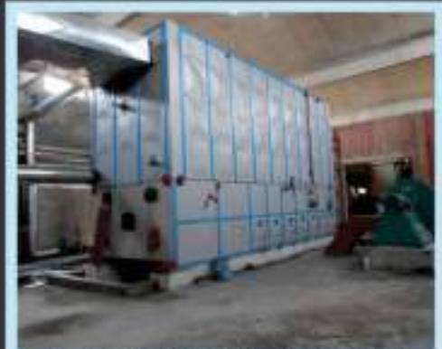
Kamal Textile Mills Faisalabad, 09 Mkal Coal Fired Thermal Oil heater
