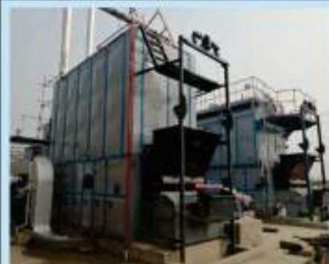
Lahore Fashion, Coal Fired Steam Boiler and Thermal Oil Heater
