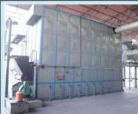
Barkha Textile Faisalabad, 08 MKCal Coal Fired thermal Oil heater
