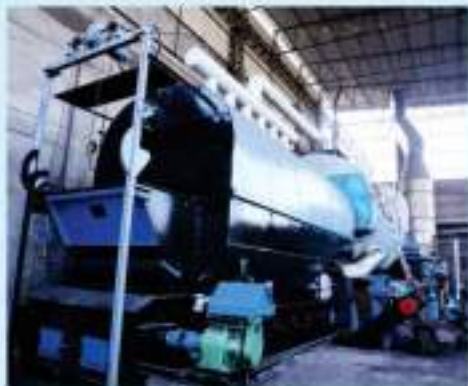
Al Ameen Moon (15 TPH Converted Chain Grate Coal Fired Steam boiler)
