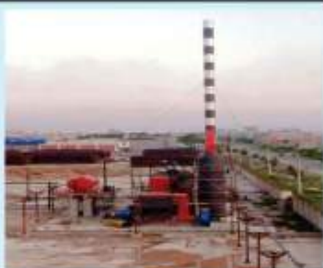
Asia Feed Mills, Biomass Fired Chain Grate steam boiler
