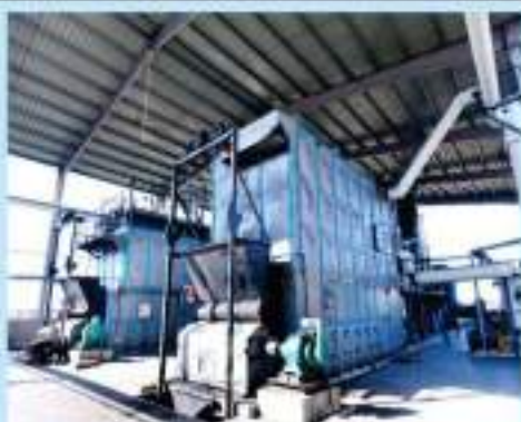
Maheen Textile (10 TPH Coal fired steam boiler & 05 Mkal Combo Oil Heater)
