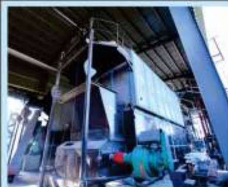
JK Spinning Faisalabad (10 TPH Coal Fired Chain Grate steam Boiler)
