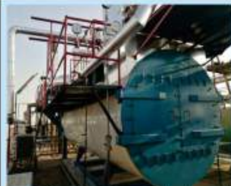
West Point Home Bahrain Triplex Waste Heat Recovery Steam Boiler
