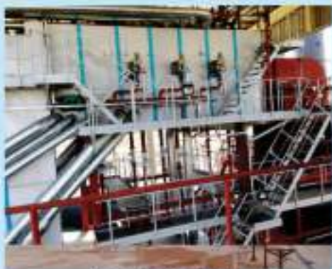
KAPCO Kot Addu 25 TPH Coal Fired Steam Boiler
