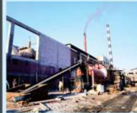
ARC Textile (Biomass Conversion of steam Boiler)
