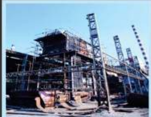
Sapphire Ferozwatwan Biomass Conversion of Chain grate Coal Fired steam boiler
