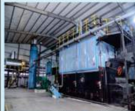
Al Makkah Textile (15 TPH Coal Fired Chain Grate Steam Boiler)
