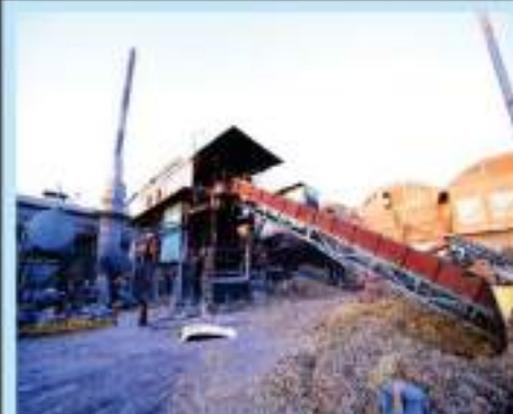
Magna Textile (Biomass Converted Coal Fired Chain Grate Steam Boiler)
