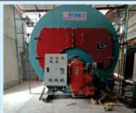
Captain PQ Chemical Karachi, 04 TPH Gas fired steam boiler
