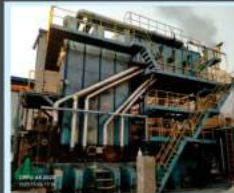
Century Paper Mill Jambar, 25 TPH Coal Fired Steam Boiler
