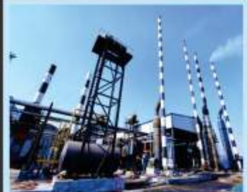
Sadaqat Limited Faisalabad (06 Nos Boilers & Oil Heater in one Shed Supplied and installed by FBL)
