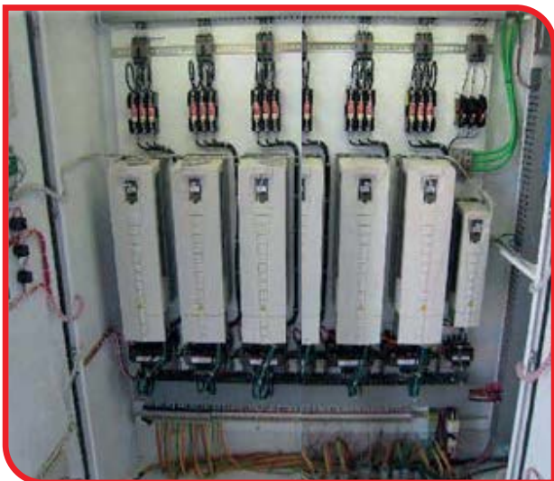
VFD (VARIABLE FREQUENCY DRIVE)
