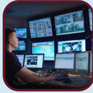
Security Control Room
