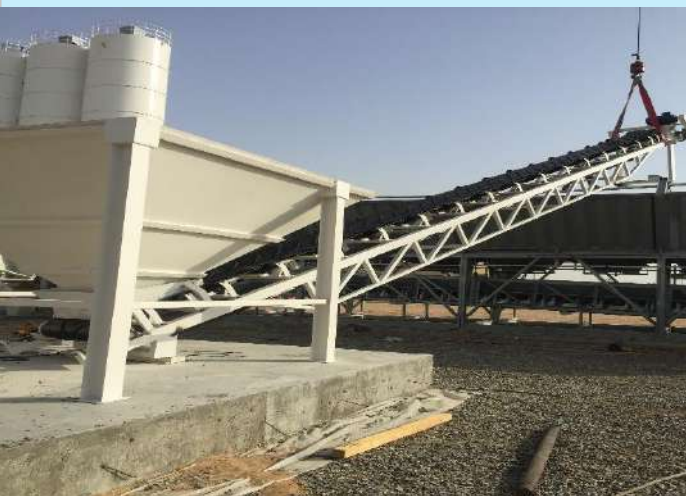
Radial conveyor belt
