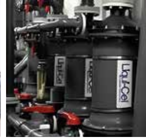
Nitrogen Treatment Services
