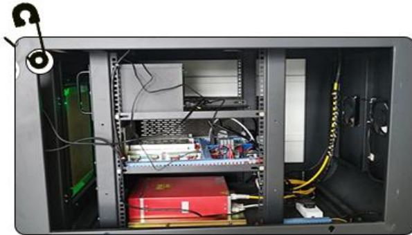
— Large capacity power distribution cabinet/chassis
