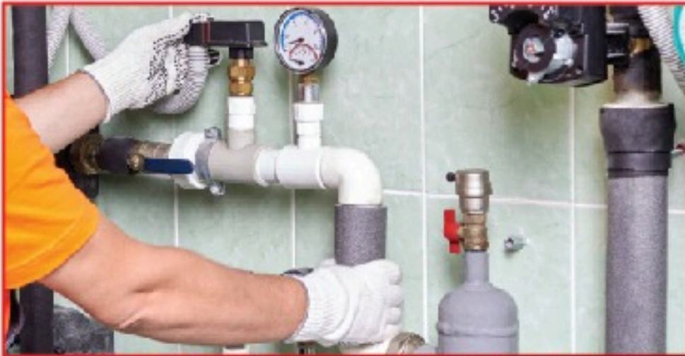
PLUMBING & HEATING SERVICES
