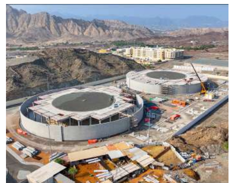
DEWA Water Reservoir in Hatta
