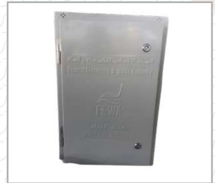
WATER METER CABINET
