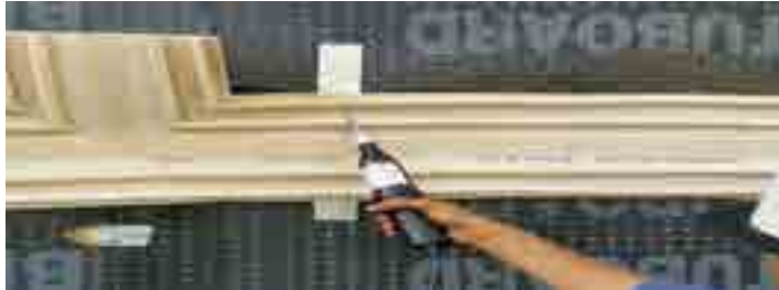
Water Bar Equipment System
