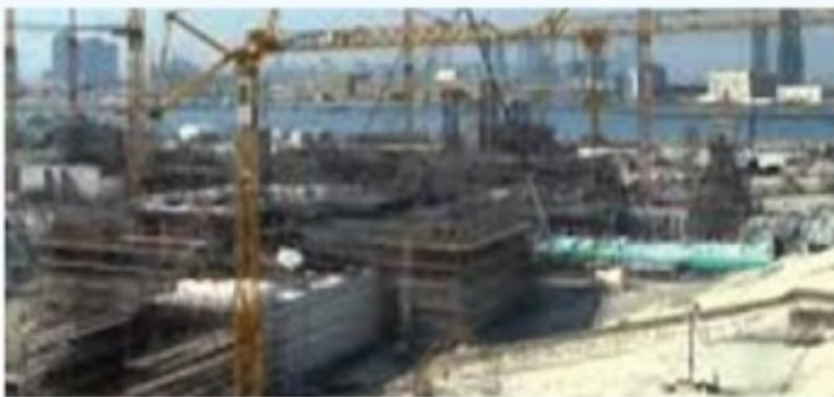
Project: Louvre Abu Dhabi Company Name: Arabtec-Sanjose-Oger(ASO). Location: Saadiyat, Abu Dhabi, UAE. Working period: From Sept-13 to July-14.
