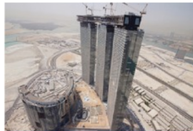
Project: ACC Gate Tower Company Name: Arabian Construction Company (ACC) Location: Al Reem Island, Abu Dhabi, UAE.
