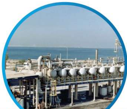
RUWAIS SULPHUR HANDLING PLANT EXPANSION (GASCO)
