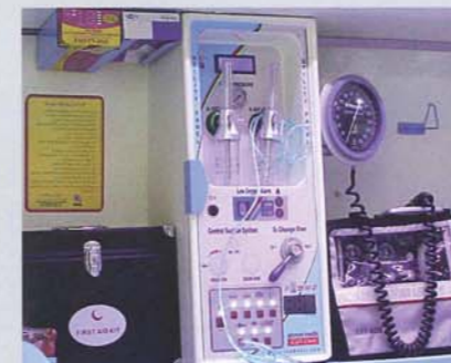
Utility Panel contains O2 flow meters, O2 cylinder changeover switch, touch panel for all switches & digital display.
