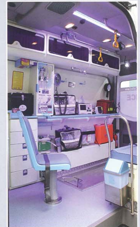
Conveniently located paramedic revolving seat, side & overhead cabinetry sufficiently accommodate all equipment.
