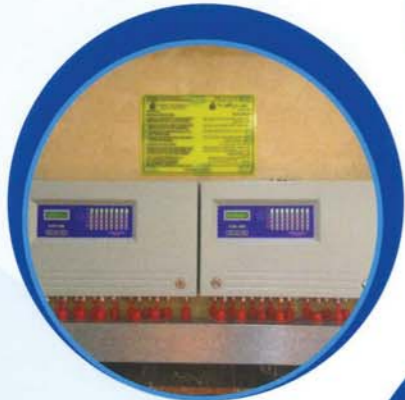
Safety Control System
