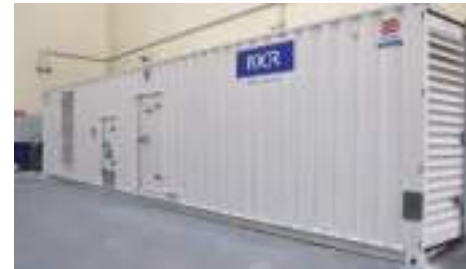
CONTAINER TYPE DIESEL GENERATOR
