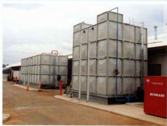
Broome Hospital, Australia
